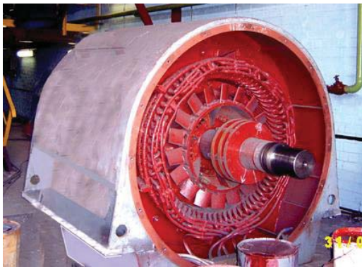
Motor: Synchronous, 1000 RPM, 10KV, 167A, 2500KW
