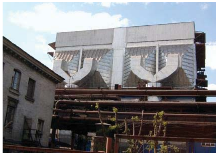
Ventilation fans of the Severstahl Steel factory in Russia, powered by 3 motors soft started by one Solcon Multi-start HRVS-DN soft starter
