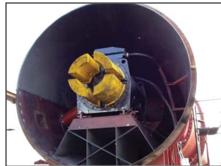
One of the 3m diameter mine exhaust fans
